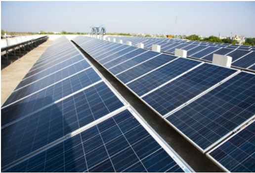
Figure 4-5 Roof Mounted Solar Panels Angled Southwards in Separated Rows
